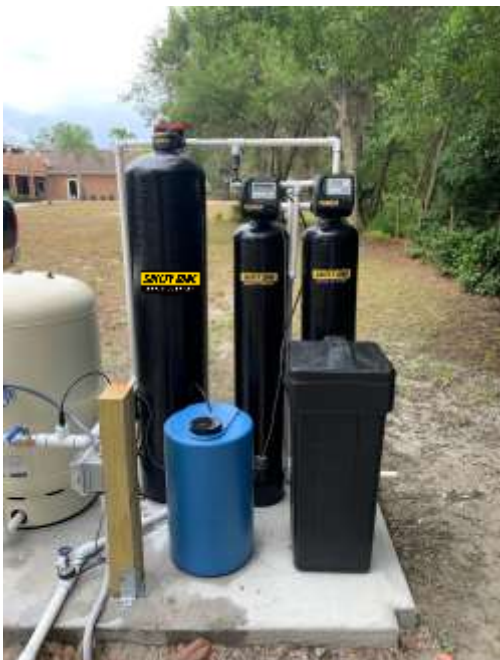
HWTP-150-1354 with 13x54 contact tank.
