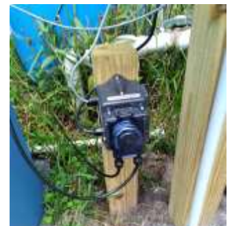
Chemical pump on post. Typical for outdoor installations.
