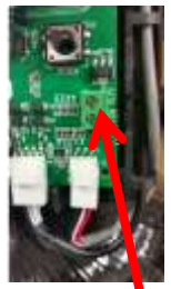
Relay connection on valve's PC board
