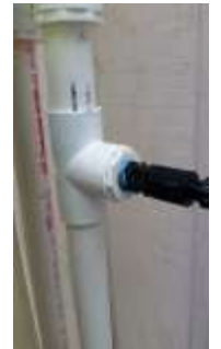
Chemical Injection Install prior to the contact tank.
