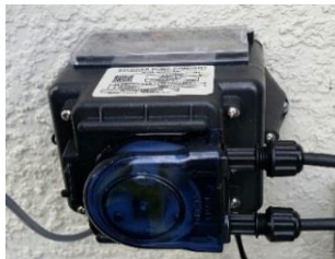
Chemical feed pump.
