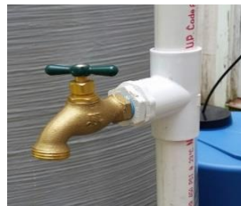
Hose bib for water sampling. (Install directly after contact tank.)
