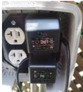
Waterproof electrical outlets are required outdoors.
