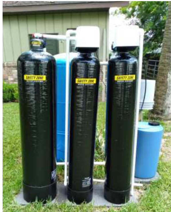
Outdoor well water installation
