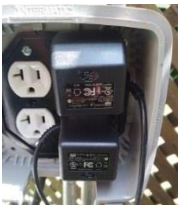
Waterproof electrical outlet needed outdoors.
